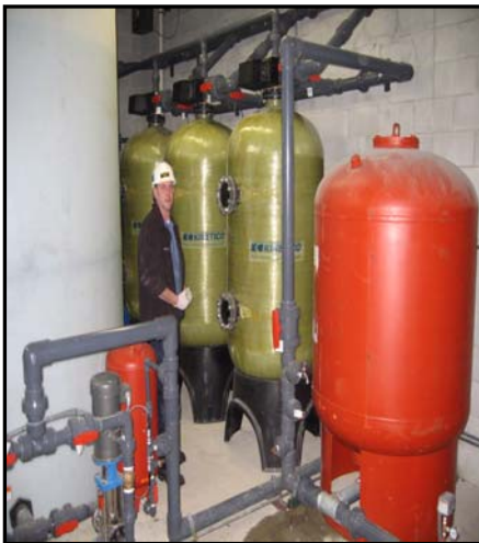
Proctor and Gamble Water Supply
